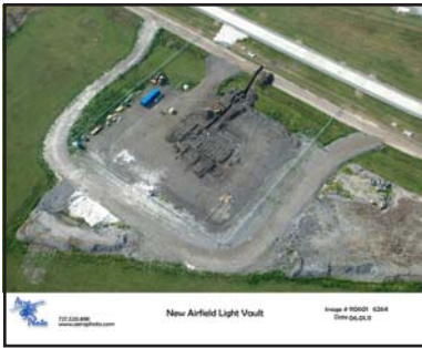
New Airfield Light Vault
